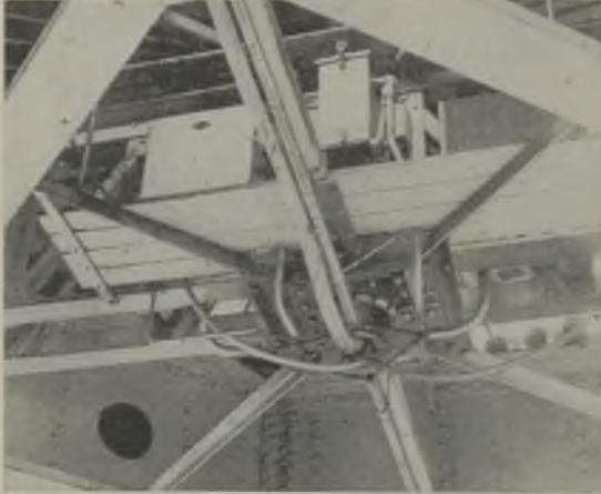
The protective panel for the travelling circuits is fitted near the centre-pin on top of the carriage; note also rotor resistance banks and lighting transformer (photographed looking up from ground)
