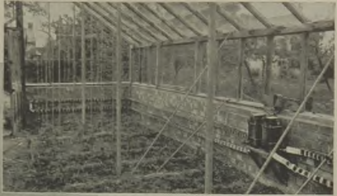
Bare elements are operated at low-voltage in this greenhouse heating scheme, so that it is permissible to use water freely
