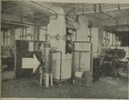
B & A Steam Boiler 150kw, supplying steam to Knitwear Presses
