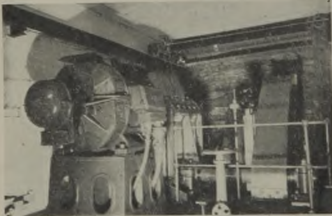
Each haulage room has an overhead crane to facilitate equipment handling
