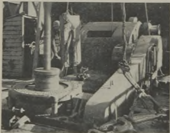
The drill pipe rises vertically through the bore hole and fits into slips in a rotary table at the base of the derrick
