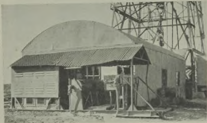
The pump and drill motor control gear is mounted on skids
