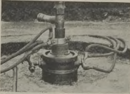
For de-waxing, positive and negative leads are connected at the well head to the production pipe and the casing, respectively
