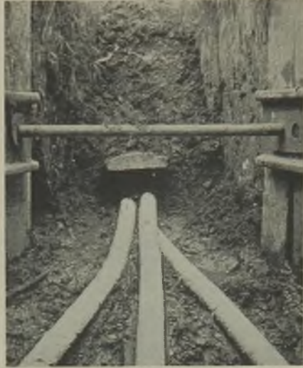
Cables trenched in triangular formation about 3 ft. deep with concrete slab protection
