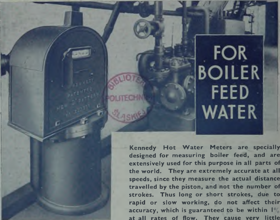
A KENNEDY POSITIVE FEED WATER METER INSTALLED ON BOILER PLANT.
