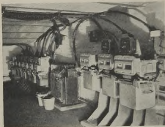
The main underground substation is about 150 yards from the pit bottom; the shaft cables connect direct to the 3.3-kV switch-gear at the far end
