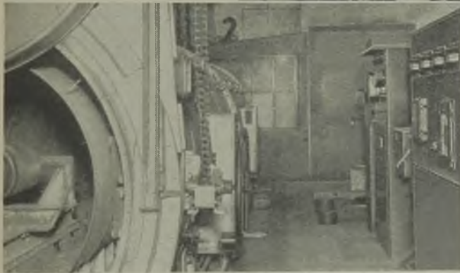
The four banks of heaters serving the heating zones of the furnace are separately controlled by indicating-type controllers, each of which is fitted with a scale for setting purposes only and is operated from a time-temperature programme controller
