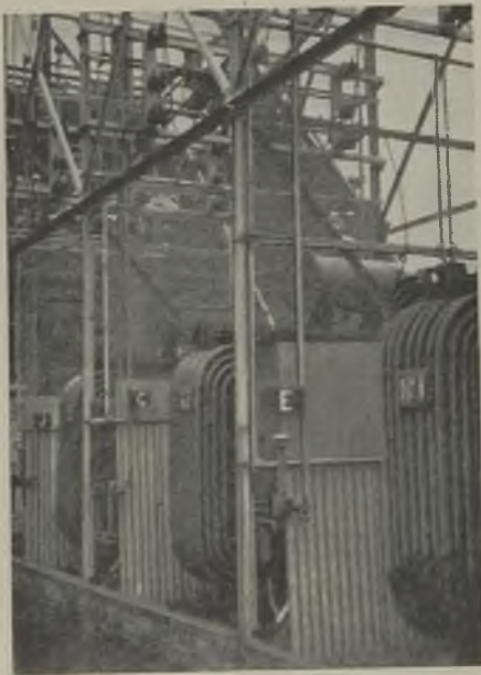
These 3.3/22-kV step-up transformers at Carmarthen substation feed the main h.v. network
