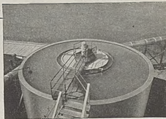
Typical ACCELATOR installation. This unit softens 2.2 million gallons of water daily.
