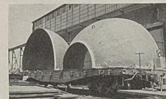
Only four welds were required to assemble the two sections of the tower head in the field.
