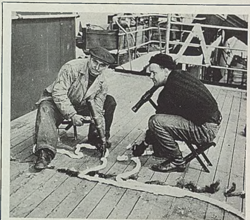
WOOD DECKS COME BACK: Workers at Federal Shipbuilding & Dry Dock Co.'s Kearny, N. J., yard drive cotton into the fir planking preliminary to caulking to make peacetime decks of the AFRICAN STAR waterfront. During the war the steel decks were not covered, but fleet operators say wood decking will add to the comfort of crew and passengers during peacetime runs
