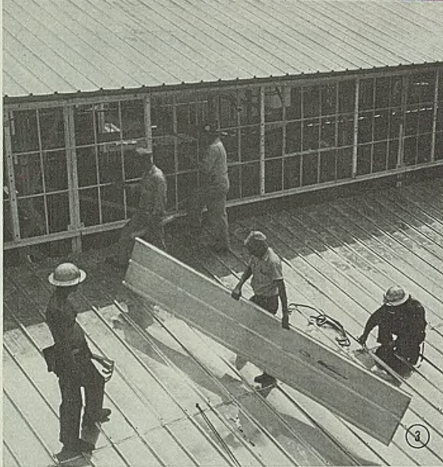
Fig. 3—Aluminum roofing on a large industrial building. Recommended method erecting the roofing panels is indicated in the following illustration
