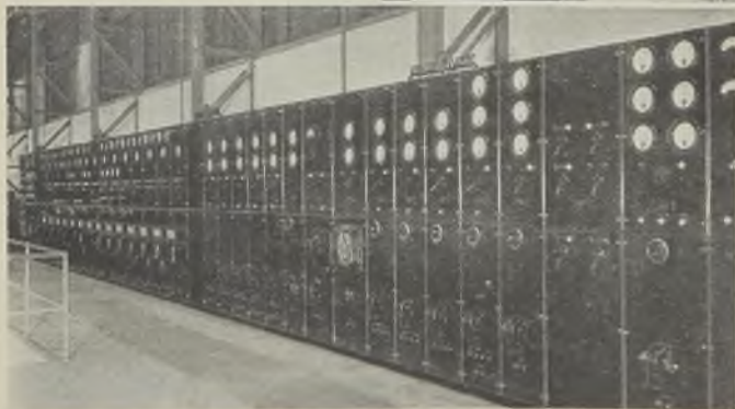
The cubicle type main supervisory board for the entire mill is about 90 ft long
