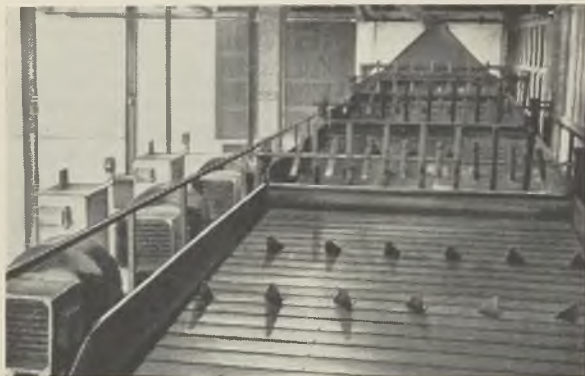
Drying tables with the fan inlets incorporating heating elements on the left
