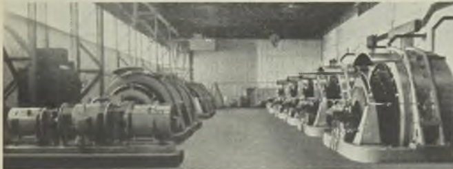
All the finishing stands are driven by d.c. variable-speed motors (right) supplied by two m.g. sets (left), each with two 2,500-kW generators
