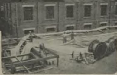
Cabling at Southwick Generating Station.
