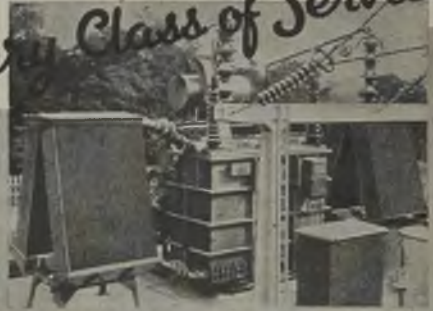
15000 K.V.A. 132,000/11,000 volt 50 cycle 3-phase G.N. Outdoor Transformer with "On Load" tap-changing gear in service on the British Grid.
