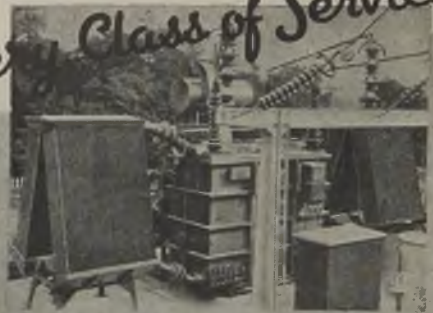
15000 K.V.A. 132,000/11,000 volt 50 cycle 3-phase O.N. Outdoor Transformer with "On Load" tap-changing gear in service on the British Grid.
