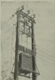
Aeroflex Cross Arm type Line Fuses protecting the L.T. side of a pole-mounted Transformer.
