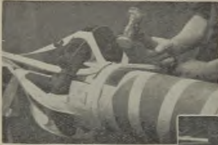
In winding a l.v. coil, a shaped press-board end piece is first applied . . .
