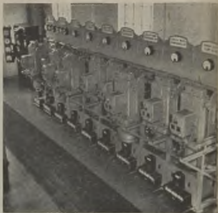
By means of section switches on the h.v. board at Westwood the three power stations—Addiewell, Westwood and Deans—can be fed to or through either of the busbars via the station interlinks
