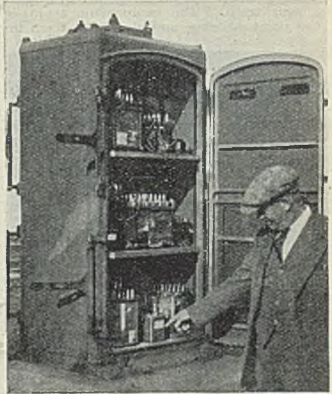
Inspection of the condenser, carried out at regular intervals, is facilitated by the simplicity in design of the equipment
