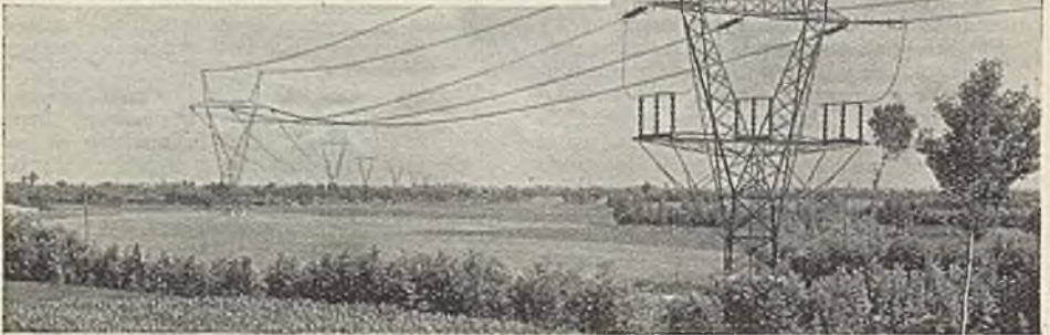
Dead-end tower at River Po crossing of 230 kV power line in Italy. The overall height of the tower is 30 m., and at the conductors 22 m. The weight of the tower is 8 400 kg.
