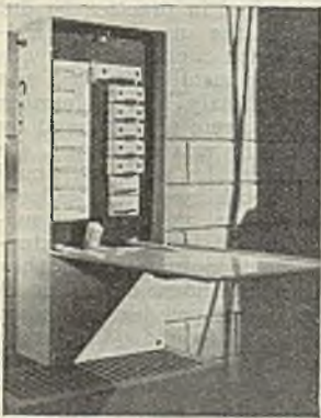
Hartley mains control unit, with servicing door open
