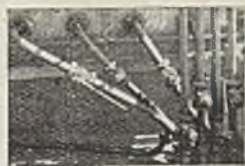
A typical 'Audco' Installation at a Chemical works.
