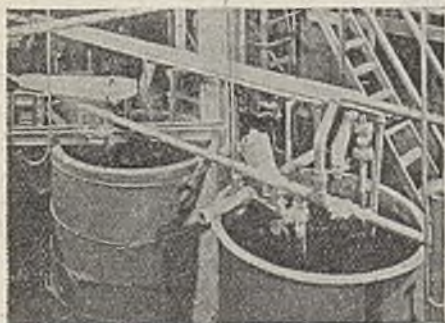
Fig. 1. Lead-lined neutraliser (left) and evaporator feed tanks. The agitator is made of stainless steel.
