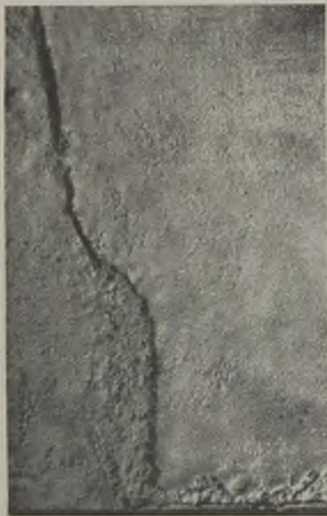
FIG. 12.—DEFECT CAUSED BY TOO HARD RAMMING.
