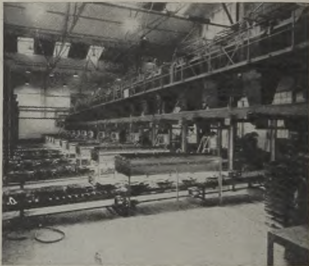
FIG. 1.—G.E.C. INFRA-RED LAMP HEATING UNITS INSTALLED IN A FOUNDRY. THIRTY-EIGHT UNITS ARE USED FOR DRYING VARIOUS TYPES OF MOULD.
