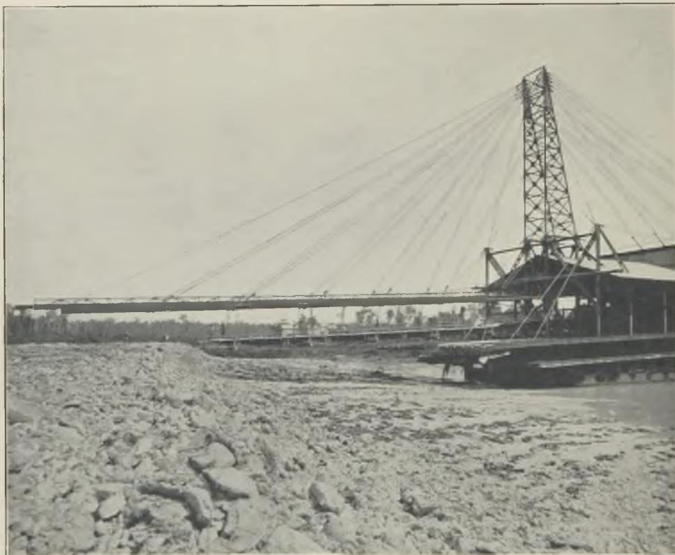
FIG. 3.—STERN VIEW OF DREDGE, SHOWING OVERBURDEN CHUTE AND LONG TAILINGS DISCHARGE PIPELINE. THE HONGKONG DREDGE CAN BE SEEN WORKING IN THE DISTANCE.
