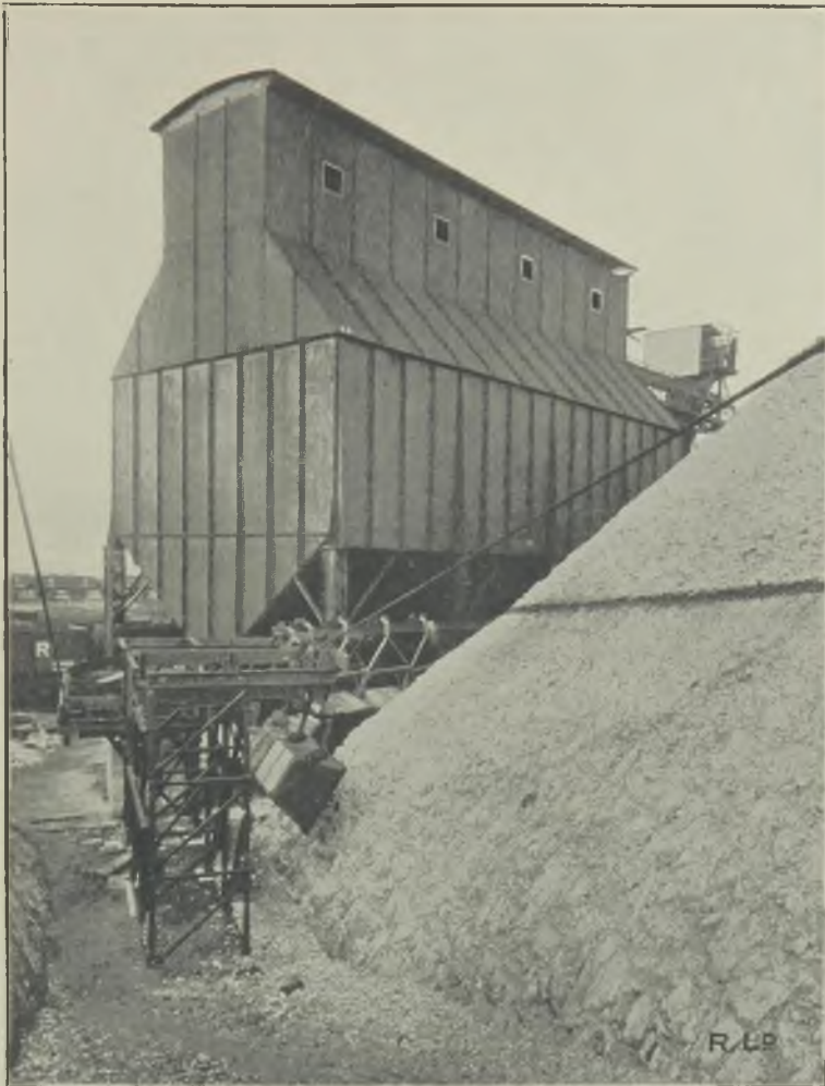
TILMANSTONE ROPEWAY.—LOADING STATION AND BUNKER.
