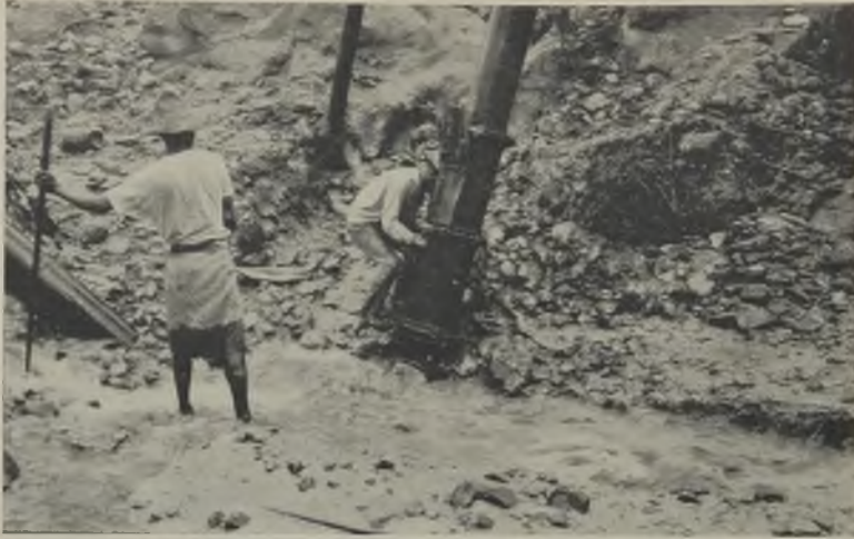
HYDRAULIC ELEVATOR IN OPERATION.
