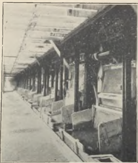
FIG. 15.—600 STAMP MILL: MORTAR BOX FLOOR.
