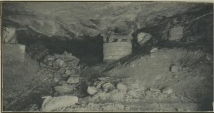
SUB NIGEL MINE—SCRAPER IN OPERATION, THE PHOTOGRAPH SHOWING METHODS OF HANGING-WALL SUPPORT.
