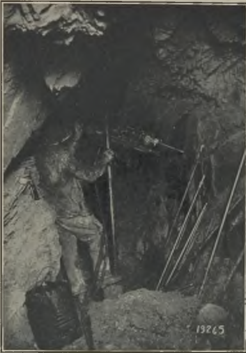
MOUNTED DRILL OF JACKHAMMER TYPE IN OPERATION AT A MINE IN IDAHO.
