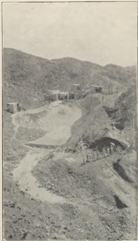
FIG. 3.—GARABIEN MINE. VIEW SHOWS EXCAVATION FOR NO. 3 SHAFT HOIST, WITH NO. 1 SHAFT HEADFRAME IN THE BACKGROUND.
