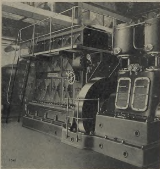
"B & M" oil engine driven air compressor.
