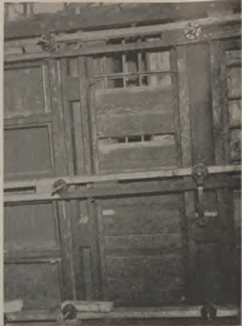
Fig. 20 — Drop - shutter forms at San Francisco permitted 12-inch lifts of concrete with good accessibility for placing shell and bulkhead concrete. Box panels (right) were used similarly in warped and tapered surfaces.
