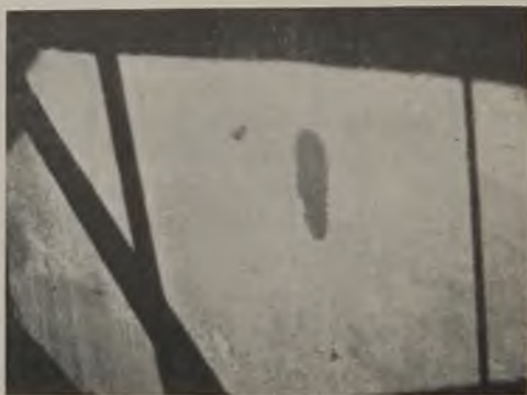
Fig. 31 —Typical minor leaks resulting from high hydrostatic test pressures with hull tanks filled with water under head 8 ft. above the deck. Even leaks like small damp spot at left of the larger spot were required by the classifying agency to be repaired, supposedly through the shell.
