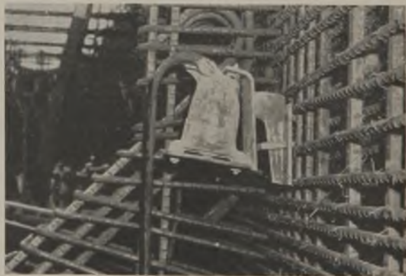
Fig. 24—Attachment used at National City with good results to apply form vibration directly to reinforcement during concrete placing.
