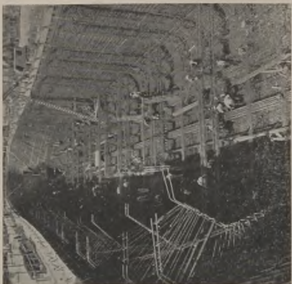
Fig. 10 (right)—Beam, bulkhead, and rib reinforcing ready for setting forms and placing first concrete in Tampa hull and beams to top of bilge.
