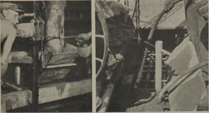
Fig. 25 (left)—Form vibrators were used effectively at Tampa on inside forms to supplement immersion-type vibrators which could not enter panels. Note method of direct placing from concrete buggies above.
