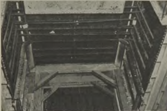
Fig. 19—Shallow-lift steel forms were placed one lift at a time as the concrete was placed at National City and provided needed accessibility for placing concrete.
