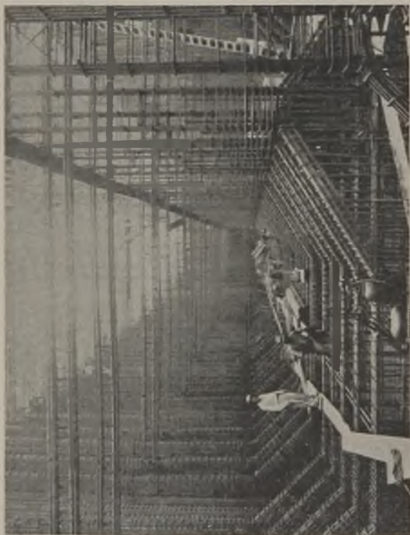
Fig. 9 (left)—Beam, haunch, and rib reinforcing in place prior to setting forms and placing first concrete in National City hull and beams to near top of haunches.
