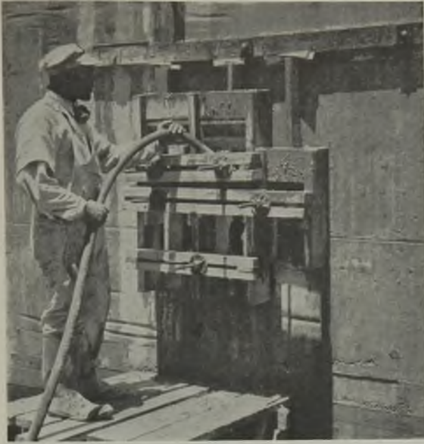
Fig. 33—After completion of concrete replacement, forms were revibrated before the concrete set and form bolts and pressure cap wedges were tightened. See Fig. 32.
