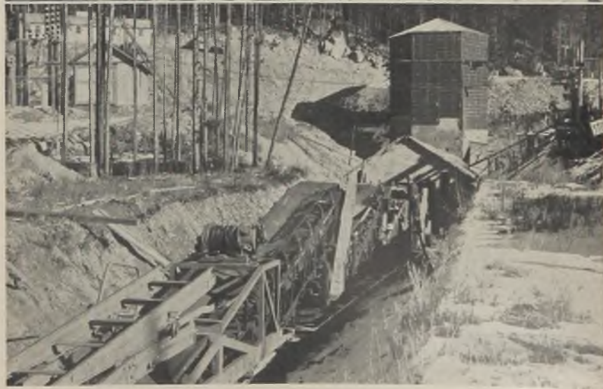
Fig. 5 (top)—The east portal batching plant was in reality two independent structures, one for the batching of aggregates and the other for the storage and batching of cement. Fig. 6 (bottom)—The west portal batching plant was erected over the tunnel portal.
