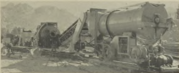
Fig. 1—The "string." Handling, mixing, and placing equipment was interconnected and traveled as a unit on the 24-in. gage tunnel track.
