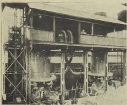
FIG. 9.—SHOWS A CUPOLA INSTALLATION BEING DRIVEN BY A KEITH-BLACKMAN FAN.
