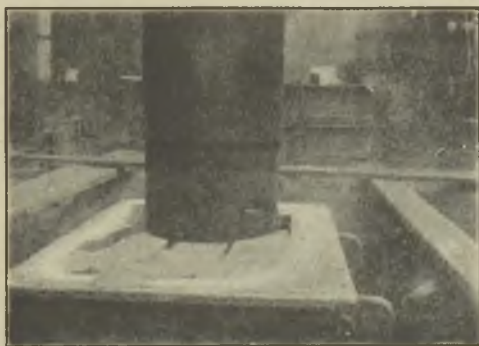
FIG. 14.—SHOWING THE MOULD IN THE PIT, WITH THE CORES IN POSITION READY FOR THE TOP PART.
