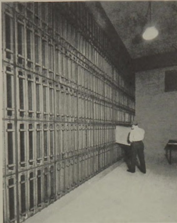
FIG. 2.—Wards Island Sewage Treatment Works, showing filters for air used in activated sludge treatment. Frame work, holders and mesh are welded and bolted Everdur sheets and strips.
