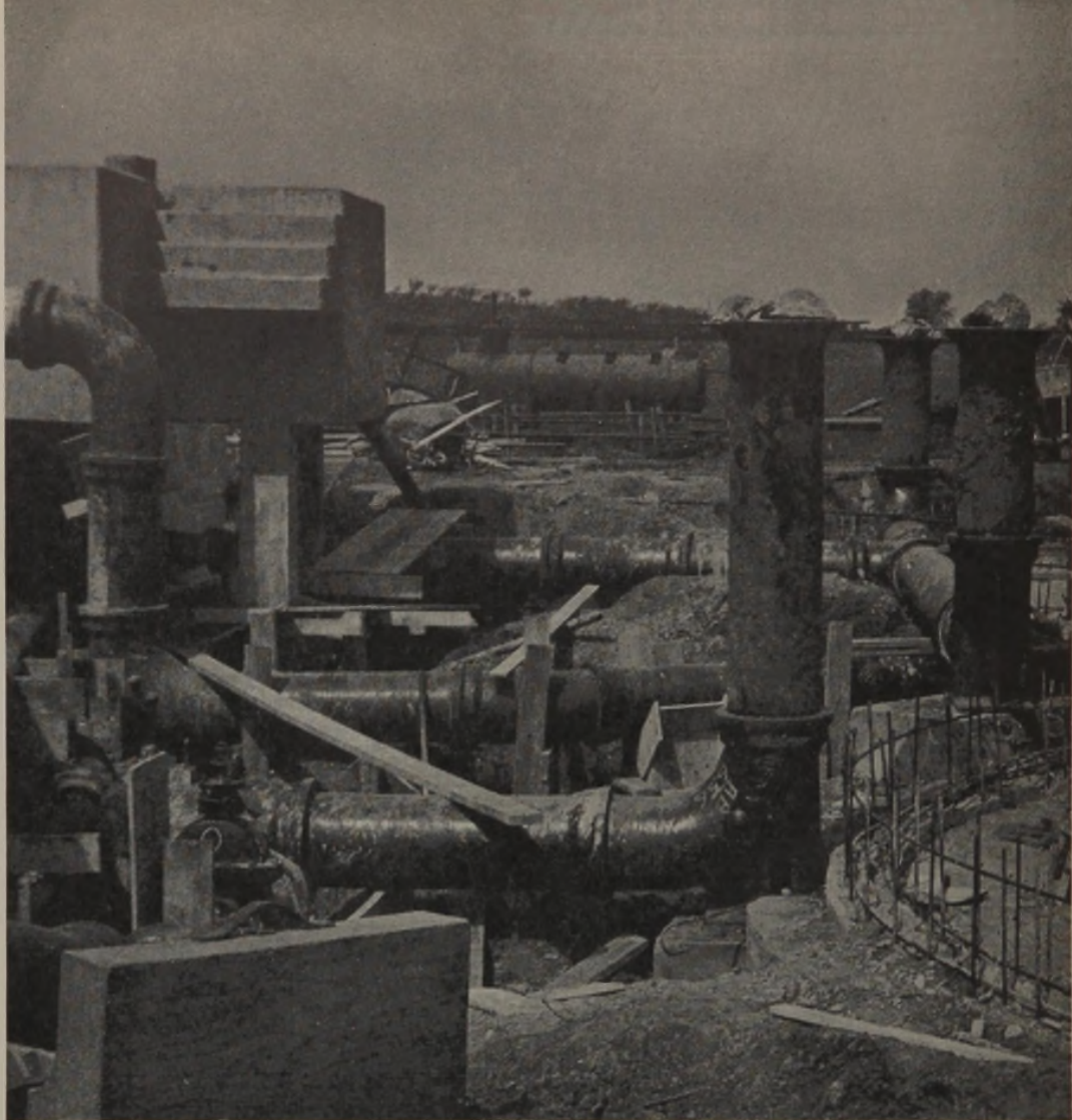
Installation of U. S. Cast Iron Pipe for Sewage Treatment Works at Winfield, Kansas
