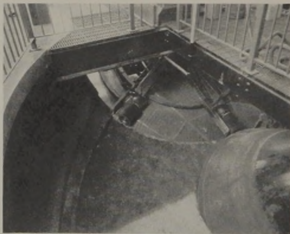
FIG. 1.—Niagara Falls, N. Y., Sewage Treatment Works, showing close-up view of one of six rotary effluent screens composed of segments of milled Everdur Plates.
