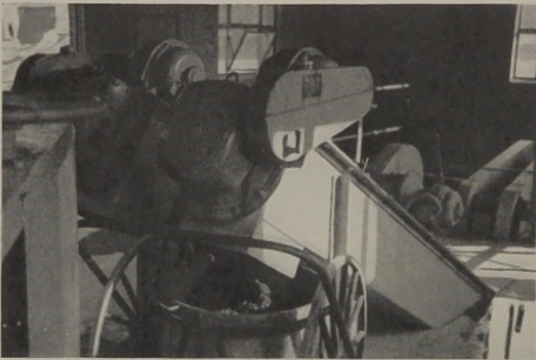
FIG. 4.—Grit receptacle mounted on push-cart affords cleanliness and minimizes odors at Danville, Illinois.
