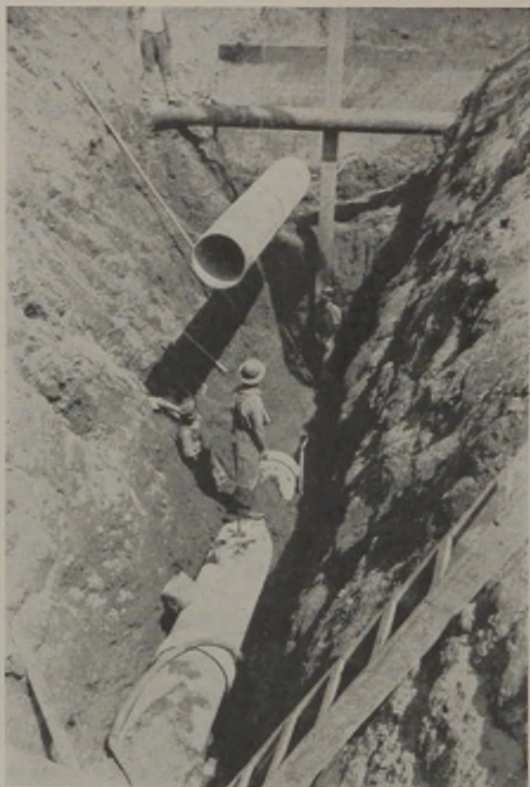
FIG. 1.—Lowering a section of large-diameter Transite sewer pipe into a deep trench.
