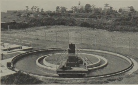
FIG. 2.—Woodbridge, N. J. Downflow magnetite filter in annular ring separate structure for straining plain settled effluent.
