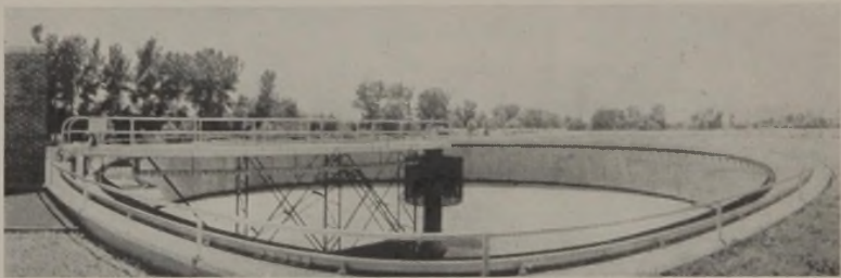
FIG. 3.—Close-up view of Link-Belt Circuline Collector in preliminary settling tank, at Quincy, Ill., showing the screw for removing scum. Engineers, Black & Veatch, Kansas City, Mo.
