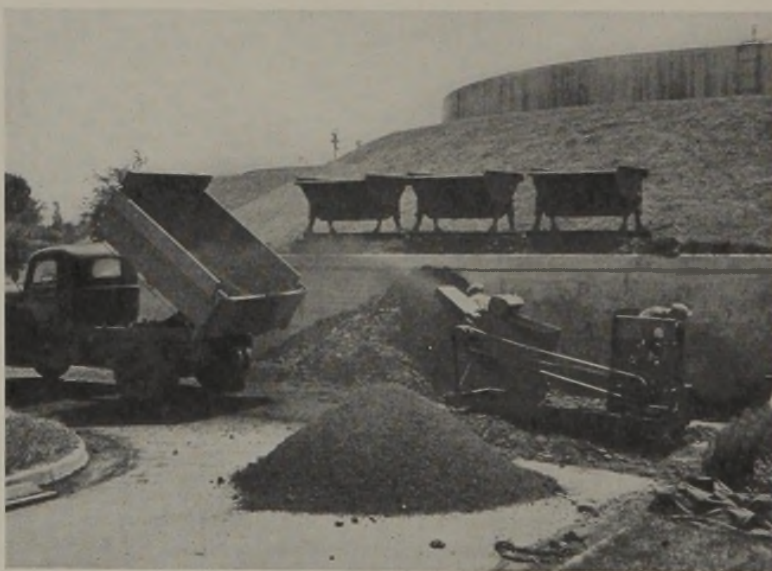
FIG. 2.—Sewage Works, Battle Creek, Mich., showing Royer "SD" stationary sludge disintegrator and product.
