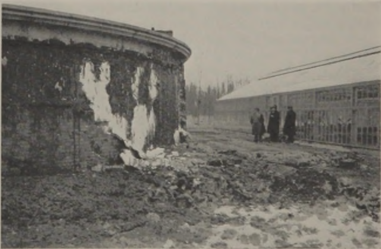
FIG. 1.—Digestion Tank “Eruption” at Sheboygan, Wisconsin, Caused by Excessive Scum Accumulation.
