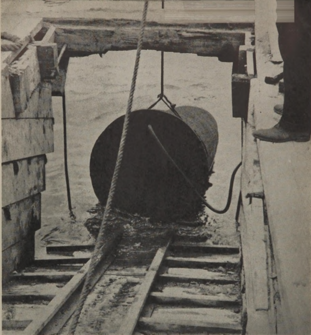
Installing U. S. Cast Iron Pipe for intercepting sewer at New Haven, Conn.
