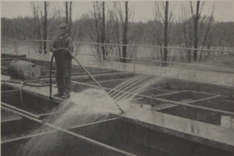
Fig. 6.—Gas Dome Scum Spray at Decatur, Illinois, W. D. Hatfield, Superintendent.
