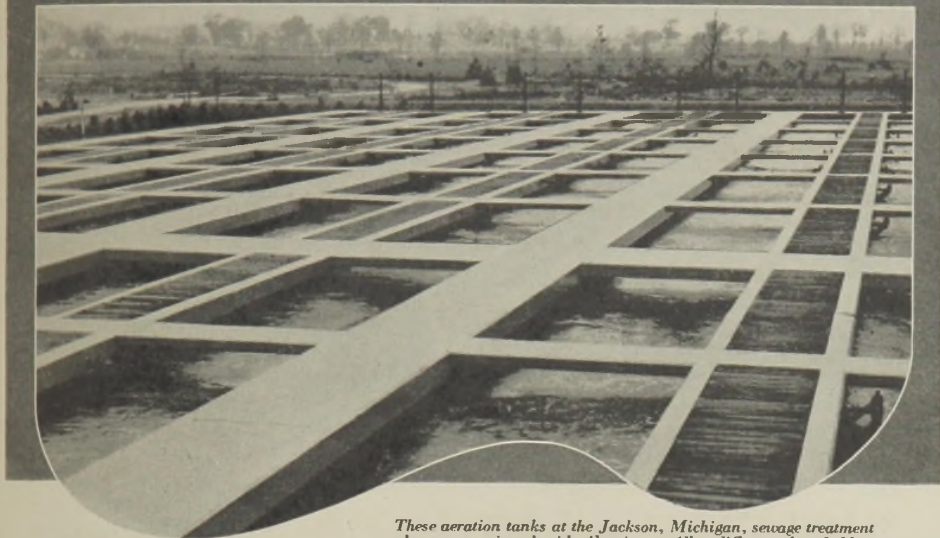
These aeration tanks at the Jackson, Michigan, sewage treatment plant are equipped with Aluminum Alloy diffuser plate holders.
