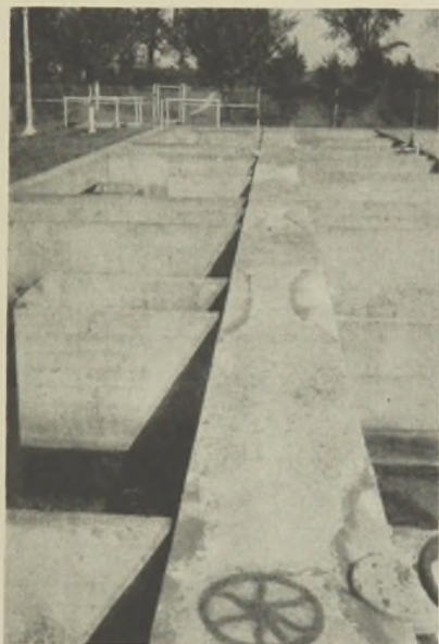
FIG. 3.—Patches after stripping of forms. Walkways pointed with cement and fine sand mixture to complete the job.
