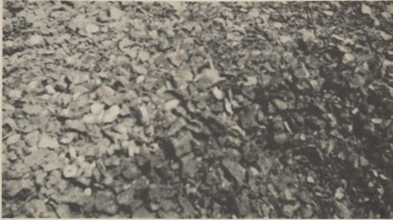
Fig. 1.—Condition of filter stone before removal and regrading.
