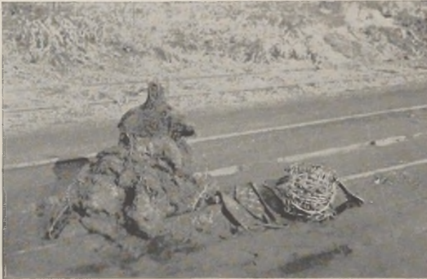
FIG. 1.—Roots and debris removed from 580 feet of 18-inch sewer. Note “drag” at right made of 15-inch root cutter wrapped with barbed wire.
