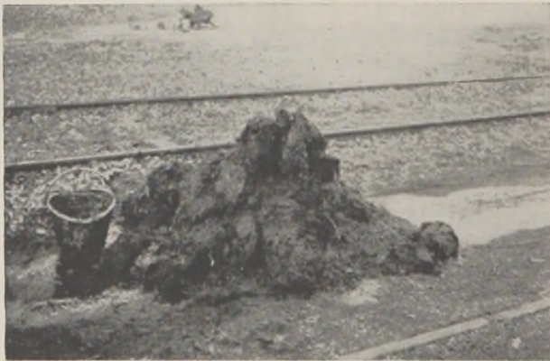
FIG. 2.—Roots removed from 300-foot section of 18-inch sewer. Bucket at left shows size of root clumps.
