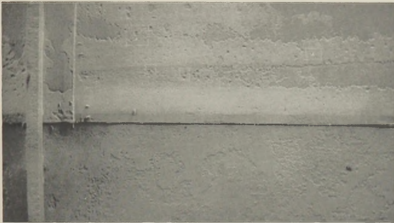
FIG. 4.—Underside of roof after sandblasting. Note pitting and holes marked with chalk.
