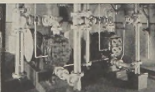
Vacuum pumps on sludge filters
