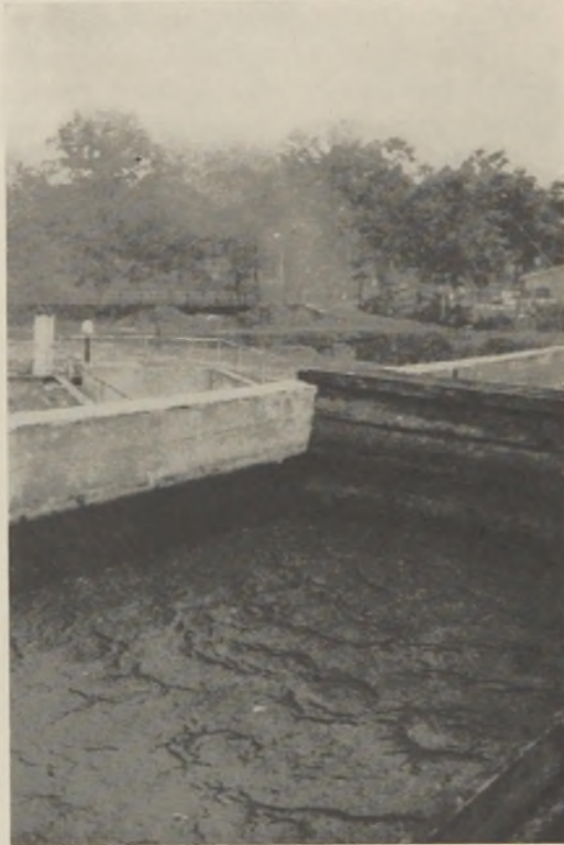
FIG. 1.—Overloaded primary sedimentation tank—a prime example of "floating sludge."
