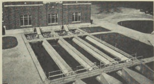
General view of 4 grit chambers employing Link-Belt STRAIGHTLINE Grit Collectors and Washers at the Joint Meeting Sewage Treatment Plant, Elizabeth, N. J.
