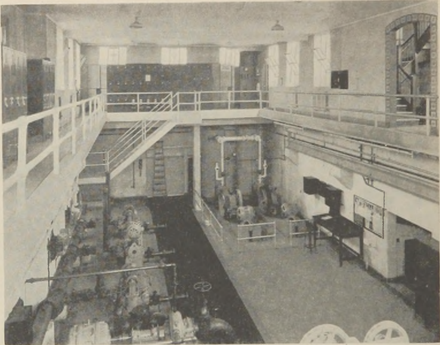
FIG. 2.—Pump room in administration building, Joint Meeting Sewage Treatment Plant.
