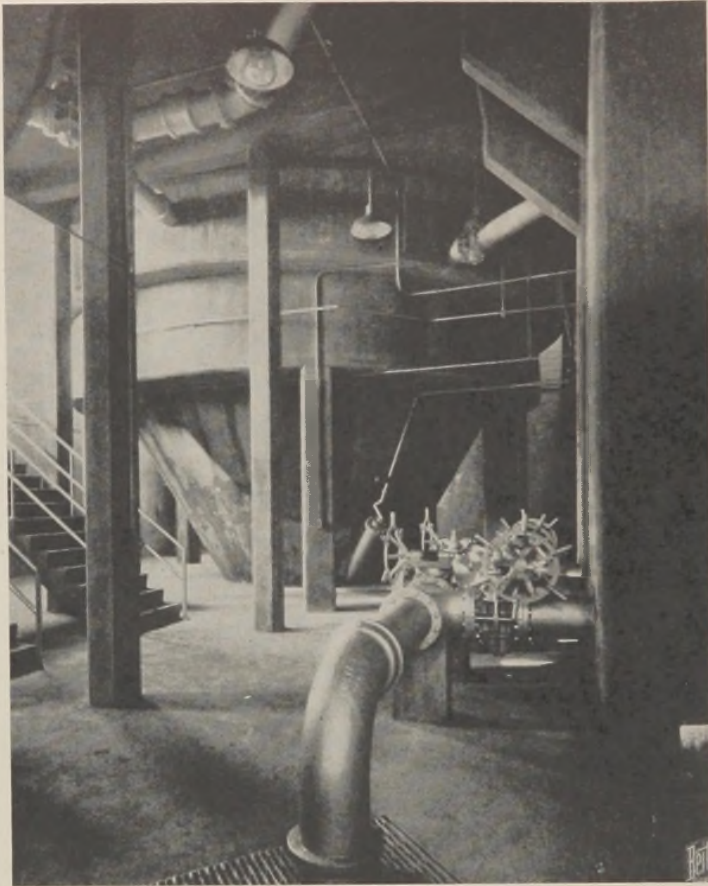
FIG. 1.—Gear-operated EMCO-Nordstrom Valves handling concentrated sewage sludge.
