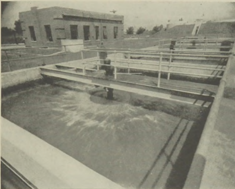
FIG. 2.—Infilco Activators at St. Johns, Overland, Mo.
