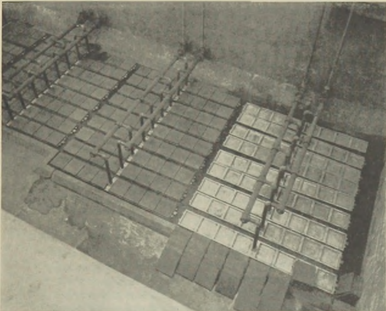
FIG. 1.—An aeration tank with aluminum diffuser plate holders at Southerly Plant, Cleveland, O.
