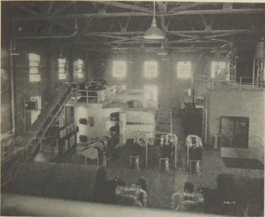
FIG. 3.—Vacuum sludge filtration and incineration equipment, Westerly Sewage Treatment Plant, Cleveland, Ohio.
