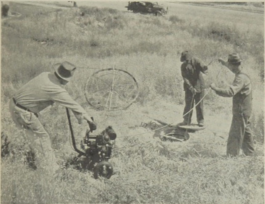
FIGURE 3.—Flexible steel rods used for sewer cleaning. Small gasoline engine power unit increases efficiency of 3-man crew.
