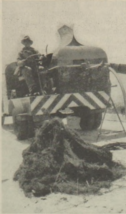
FIGURE 2.—Cleaning machine clears a bad root stoppage. Root shown is 120 feet long.
