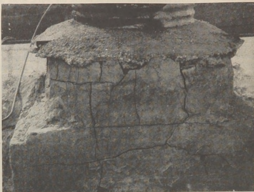
FIGURE 6.—Maintenance crews should record damage to all structures such as this manhole at which corrosive gases have been active.
