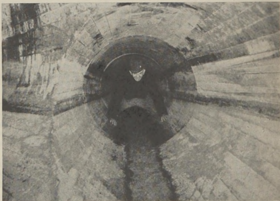
FIGURE 7.—Routine inspection is a fundamental of proper sewer maintenance. This sewer had been tested for toxic gases and oxygen deficiency to determine if it could be entered safely.
