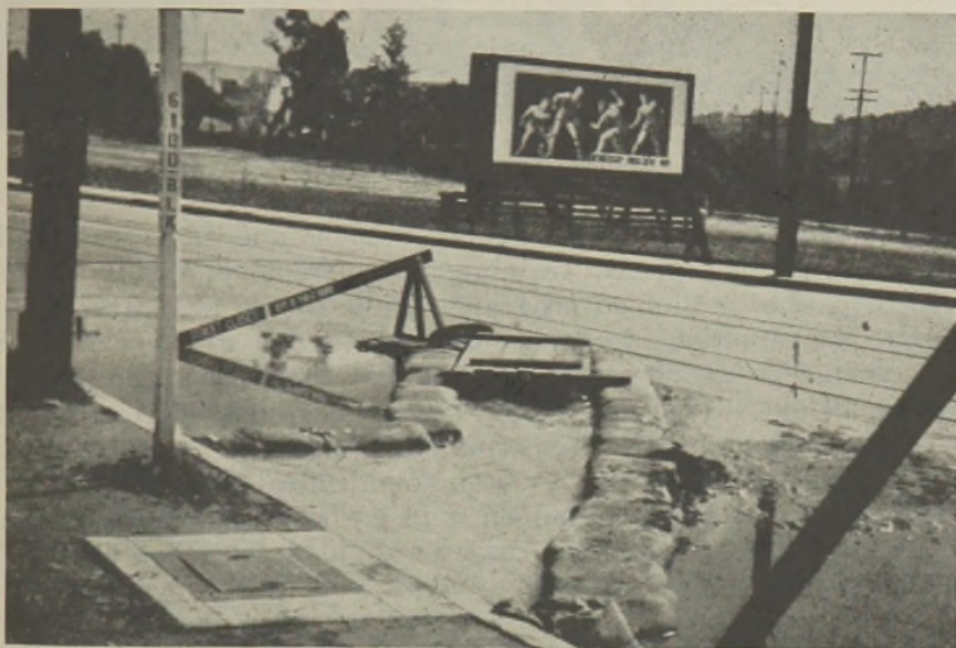
FIGURE 8.—By-passing sewage from overflowing manhole to storm water inlet while repairing broken line. Sand bags confine flow.
