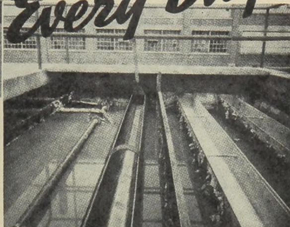
Settling Tank for the settling of coagulated wastes; showing one flight, chain, sprocket and shaft of L-B Sludge Collector; Roto-line scum skimmer; baffle board and troughs for run-off of treated waste water. Water level lowered to show equipment.
