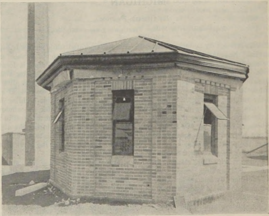
FIGURE 1.—Exterior of building damaged by digester gas explosion at Traverse City, Mich.
