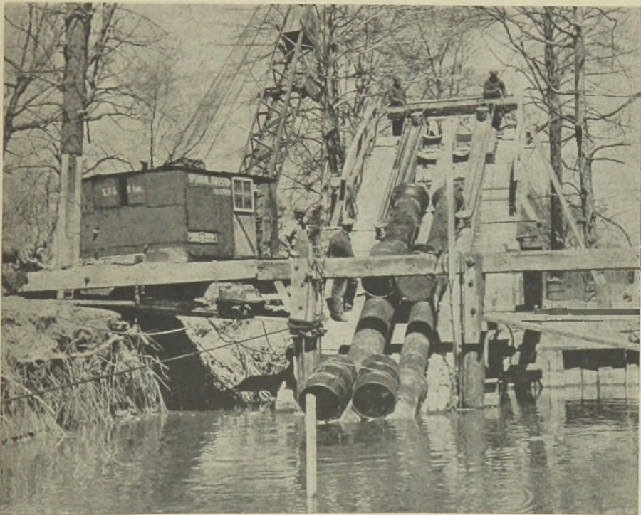
FIGURE 1.—Installing 14-in. and 18-in. flexible joint cast iron pipe for dual line sewer siphon across the Passaic River, Fair Lawn, N. J.
