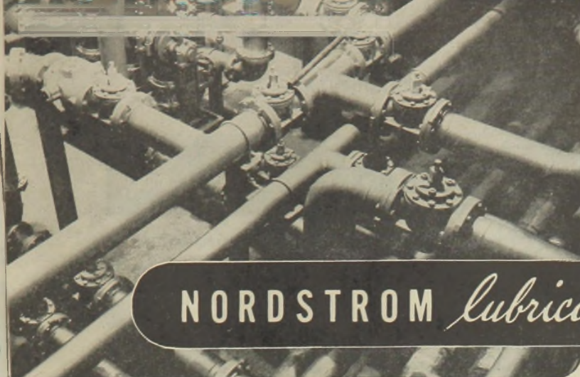
Nordstrom Valves controlling sludge lines in Greater Greenville, S. C. plant.
