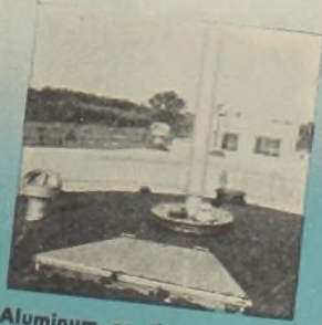
Aluminum on the roof—vent pipe, hatch cover, ventilators—all aluminum. All resistant to weather and corrosive gases.
