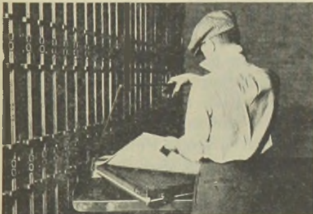
FIGURE 1.—Air filter of secondary room of the Ward's Island sewage treatment plant. Framework of filter structure and filter holders is of welded and bolted Everdur sheet and strip. Retaining mesh for filter is perforated Everdur sheet. Fabricated by American Filter Co., Inc.
