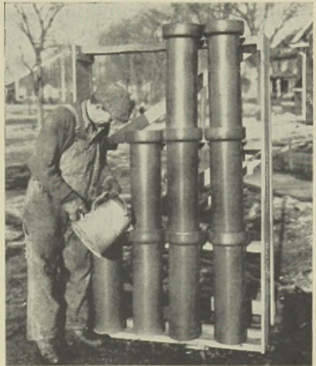
FIGURE 1.—Racks of this kind make it simple to pour several ClaPipe joints at a time in advance of installation. Pipe is kept in true alignment while pouring.
