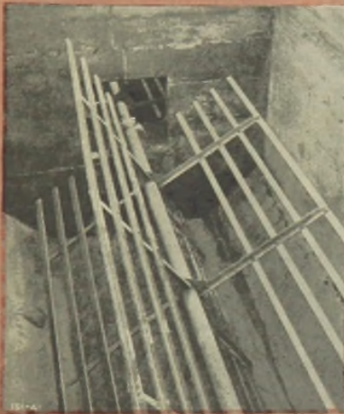
← Individual view of one of the FLOCTROLS installed in Water Treatment Plant, Newark, Ohio. Shows arrangement of compartment and paddle wheels.
