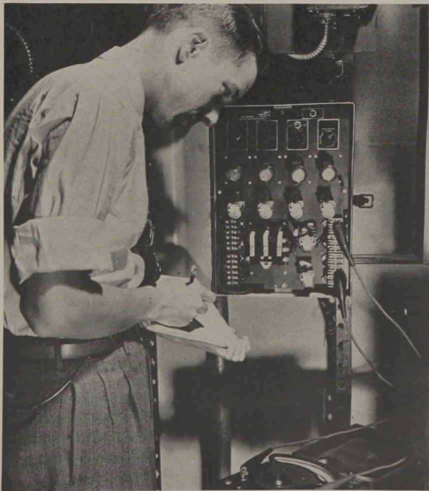
Below. Equipment should be checked to see that line voltage corresponds to panel nameplate rating, or within variation of 5% of marked value.
