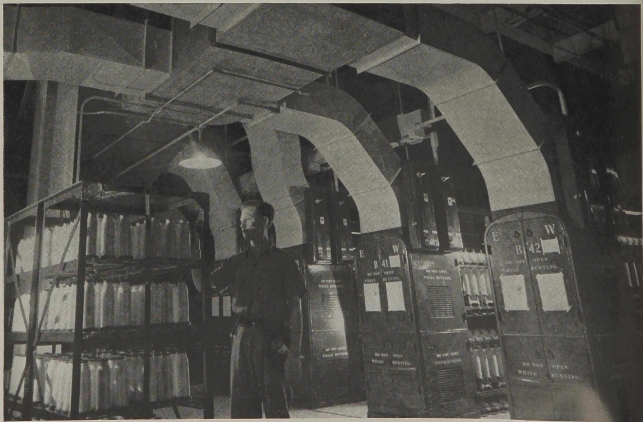
Every section of the du Pont nylon plant at Seaford, Delaware, is air-conditioned. The huge vents shown in this view provide fresh, clean air at all times.
