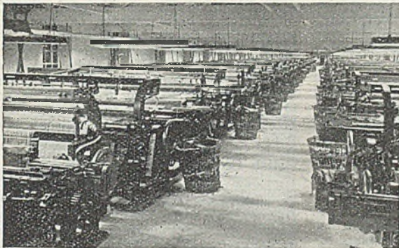
New fluorescent lighting scheme in the weaving shop of a blanket mill
